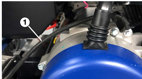
Figure 5 - Locating Negative (-) Cable
